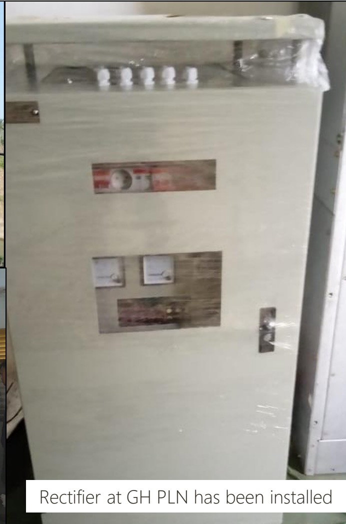
PLN Interconnection Panel 100% done
